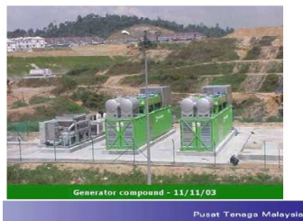
Figure 7: THS bioenergy plant
